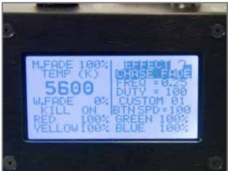
B-24 Control Ballast
